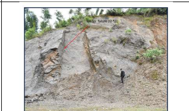
Figure 4. planar and wedge failure of RMR15
